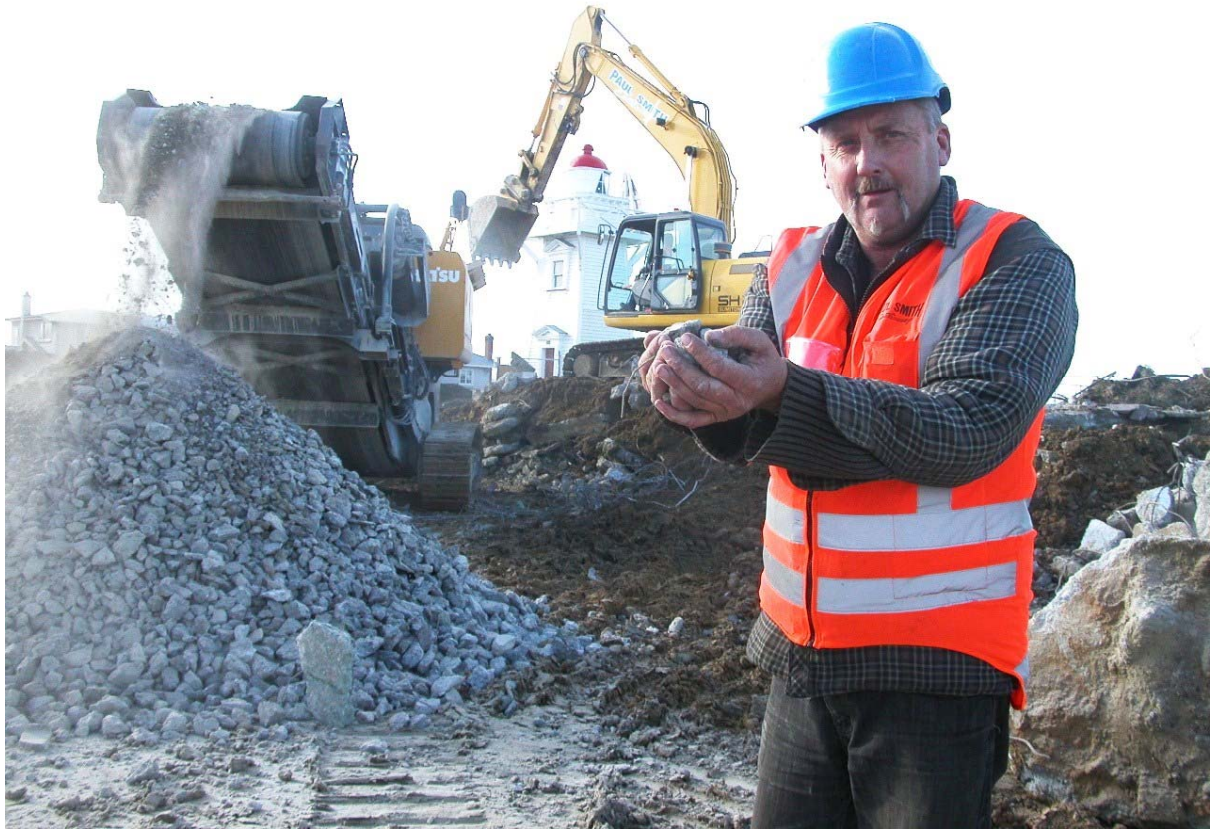
Digesting a swimming pool and producing reusable materials: Paul Smith Earthmoving machine operator Andy Smith, of Timaru, holds rubble ranging from 65mm pieces of concrete down to pebbles, the product of the company's high-technology concrete crusher pictured behind him spewing out materials suitable for recycling back into the new Caroline Bay Aquatic Centre.
