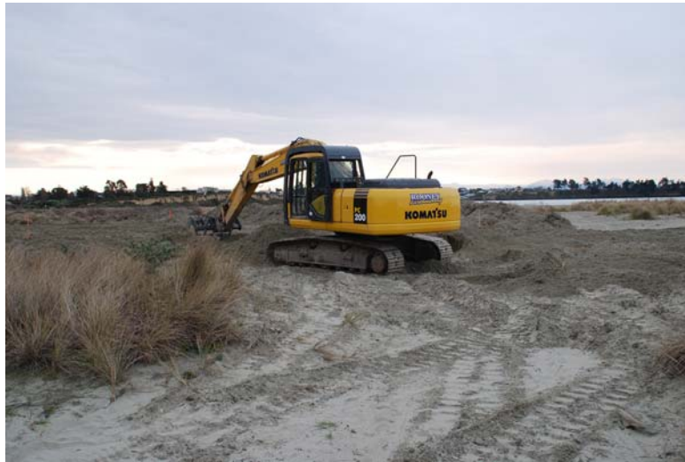
Earthmoving equipment starts work on the new carpark close to Marine Parade.
