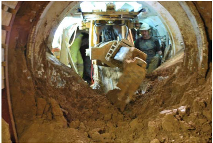
Tunnel boring machine breaks down the last of the barrier between the tunnel halves
