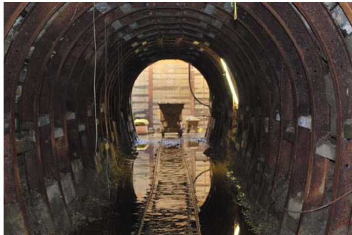
Pick and explosives used to create this part of the tunnel. Water seepage from clay
