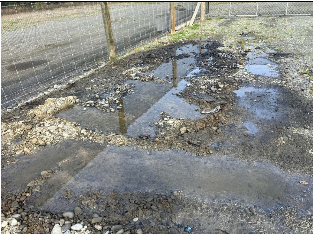
Photograph 12: Staining and debris observed (16-Apr-2025).
