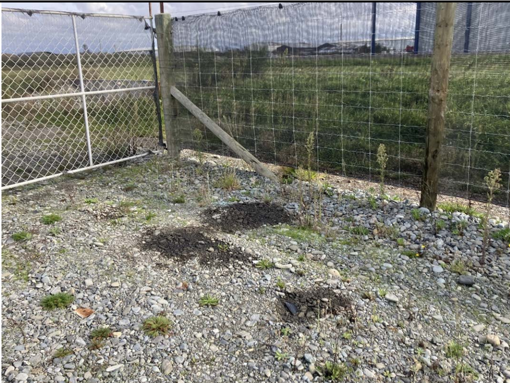
Photograph 13: Staining and debris observed (16-Apr-2025).
