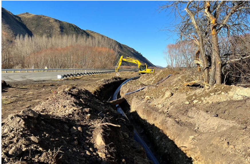
Te Ana Wai Section 2 pipeline: looking towards Rocky Gully River Crossing, going under the existing Downlands trunkmain.
