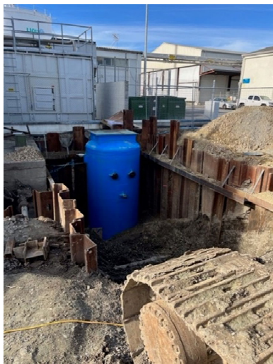
Dawson St pump station wet well.
