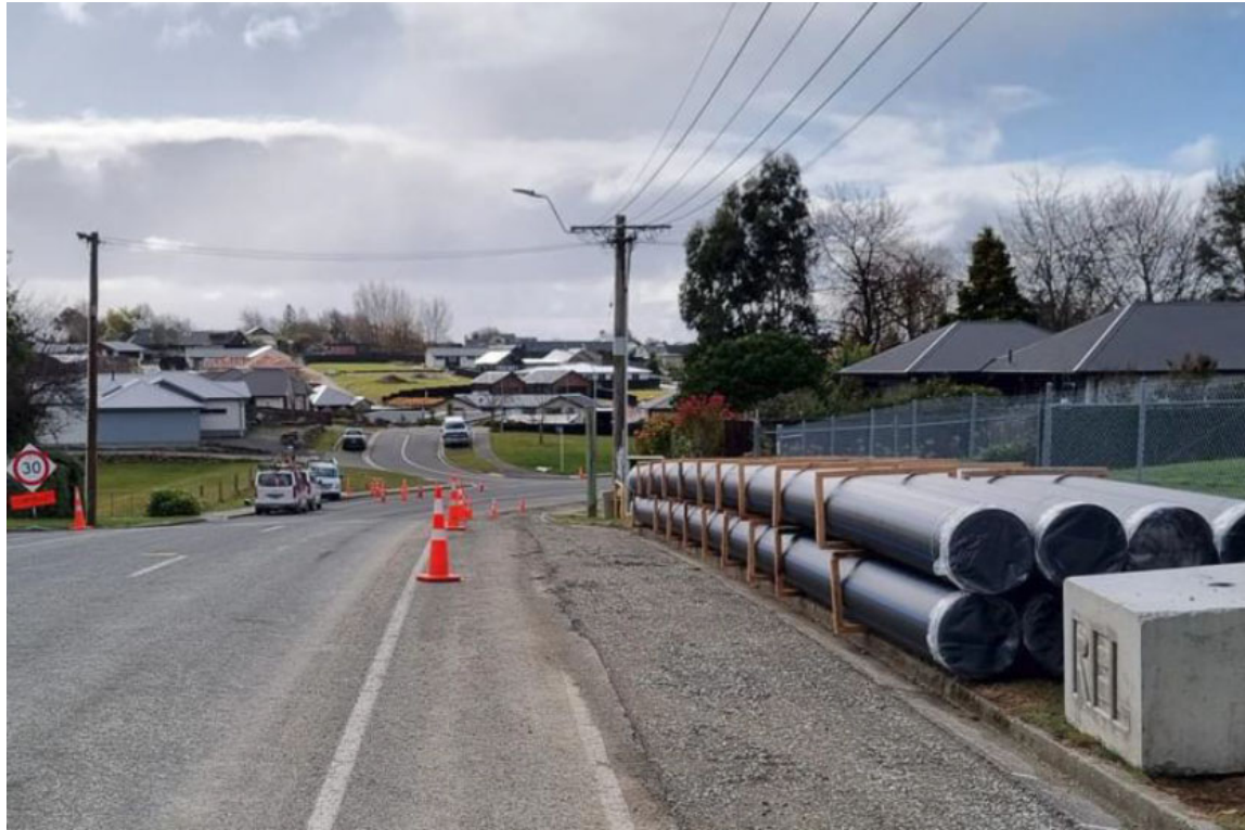
Section 2: Currently working past the S bend on Mountain View Road by Fisher Place intersection.
