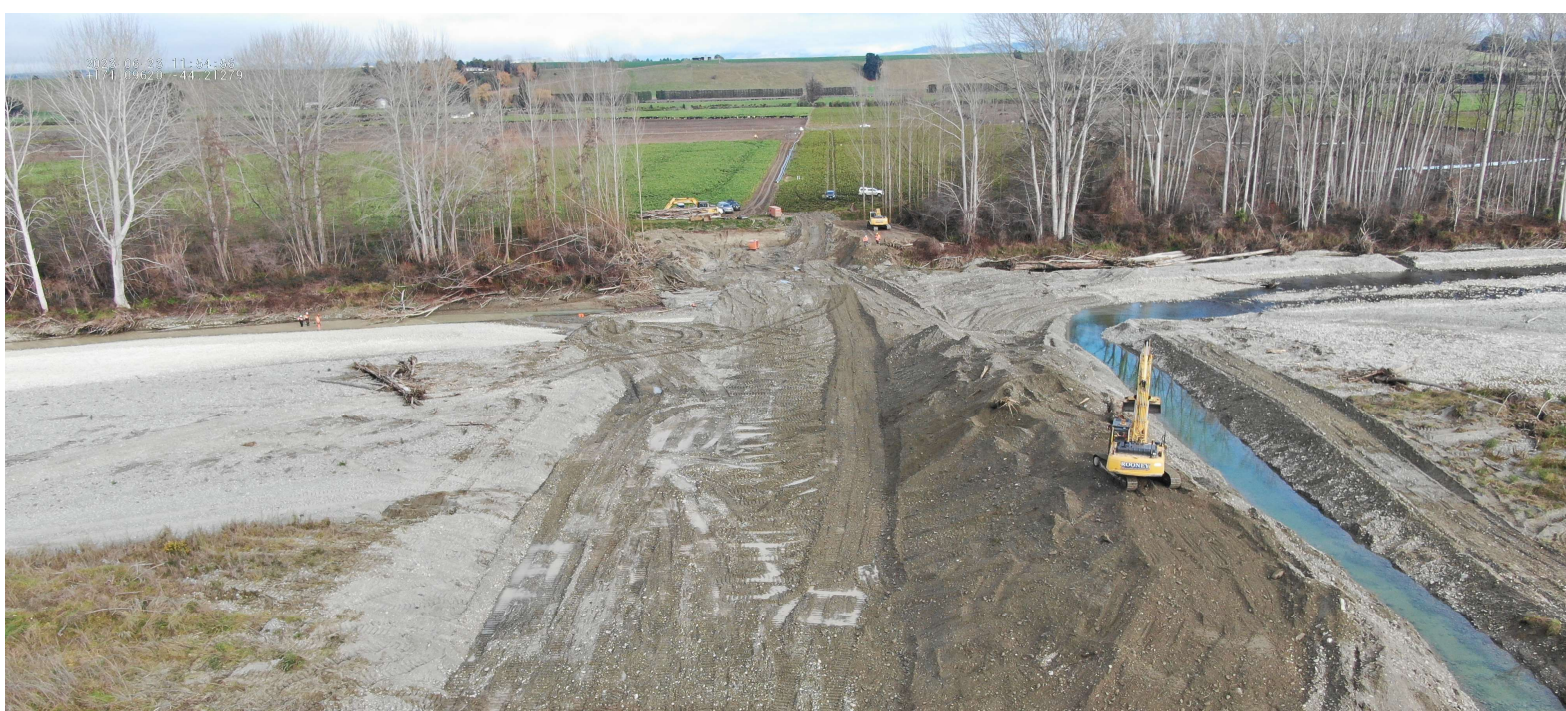
River diversion works well underway, along with fish management happening to the left of clearing.
