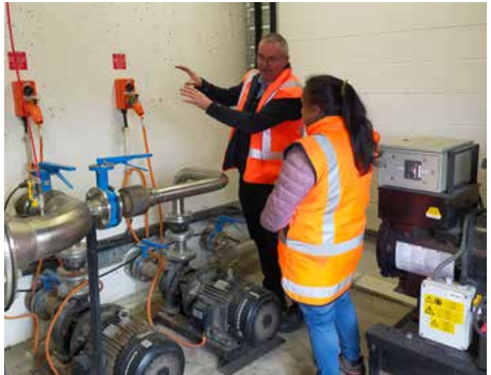
Seadown Water TP – Our Water Services Operations Engineer showing our new Three Waters Compliance Officer around the treatment facility
