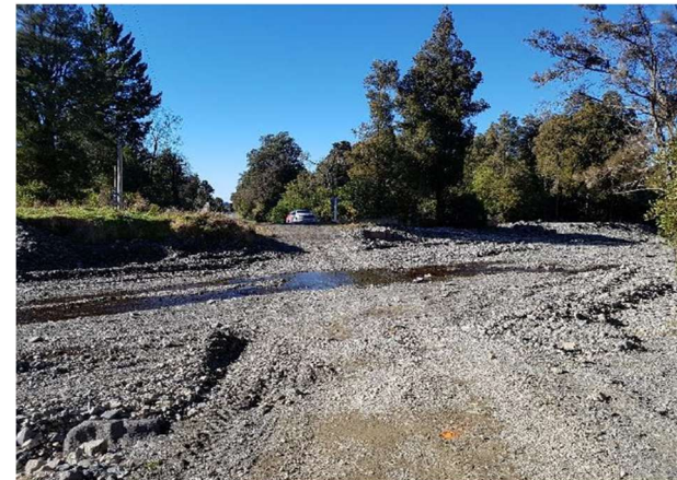
Figs. 95 and 96 (above and below): There is strong community support for an upgrade of Kowhai Stream Ford, which provides sole road access for approximately 10 properties. Maintenance requests are also frequent, diverting staff and contractor resource from other activities. Options for upgrade/level of service increases were presented to Council's Infrastructure Committee for approval in November 2023. The Committee did not agree to a level of service increase, therefore we are likely to see customer dissatisfaction trends continue at this location.
