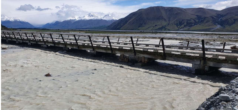
Fig 93: Forest Creek Bridge – high river flows have reduced the extent of Forest Creek Bridge, and caused significant damage to one of its piers during the 2021 flood event.
