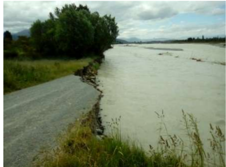
Fig. 70: Ferry Road, Arundel – During the December 2019 flood event that closed all connecting bridges across the Rangitata River and temporarily severed the South Island in two, the Rangitata River flow diverted onto road reserve and forced the abandonment of a large section of Ferry Road. In the time since this event, the river has not diverted back to previous channels and this section of road remains closed.
