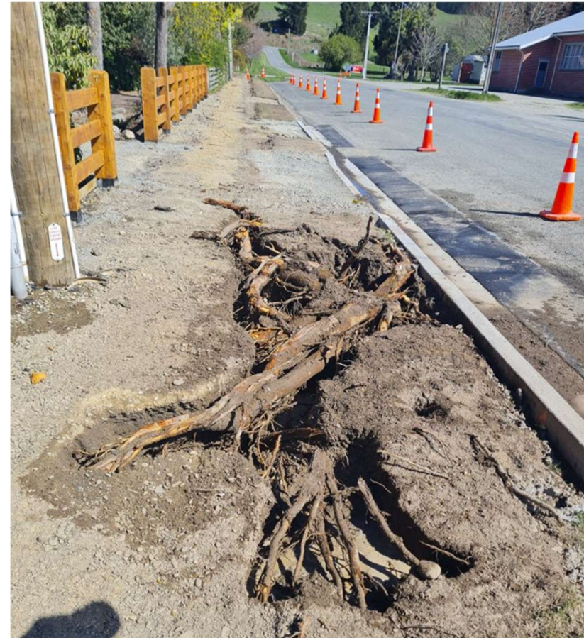
Fig. 106: Street tree damage on footpath network
