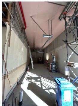
IMG_2094 - Firerating to underside floor
