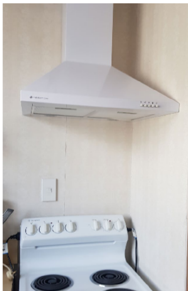
Example of installed range hood.
