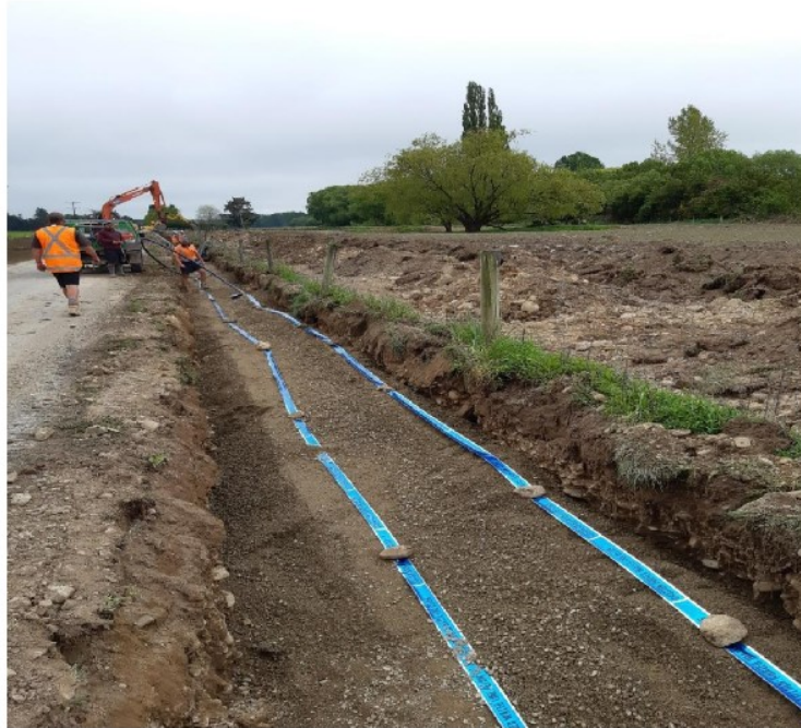
Contract 2468 – New pipe Installation both Pareora Trunkmain and ridermain in the same trench in Cliffs Road
