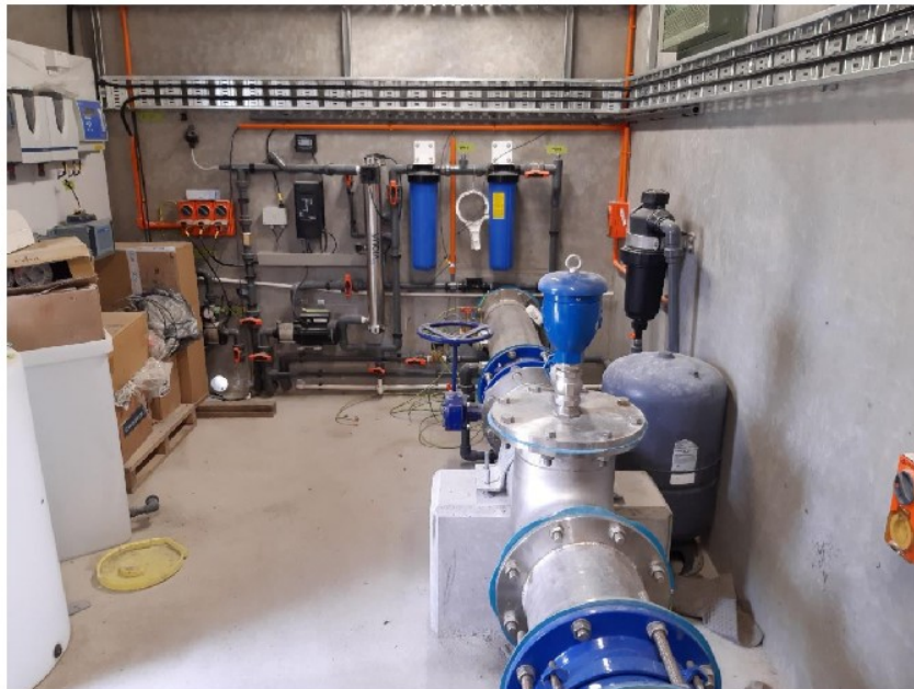
Contract 2468 – Inside a commissioned Flow Control Valve Station in Lindisfarne
