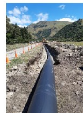
Pareora Water Pipeline Section 1
