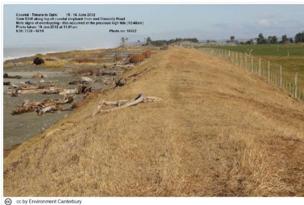
Figure 2-5: Debris left on stopbank south of Connolly road following June 2012 storm. Source: ECan.
