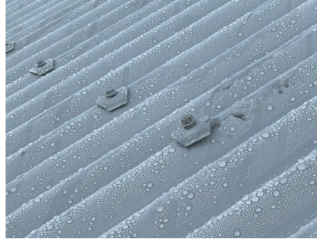
20260623_ASVR15_18 - Roof fixing review
