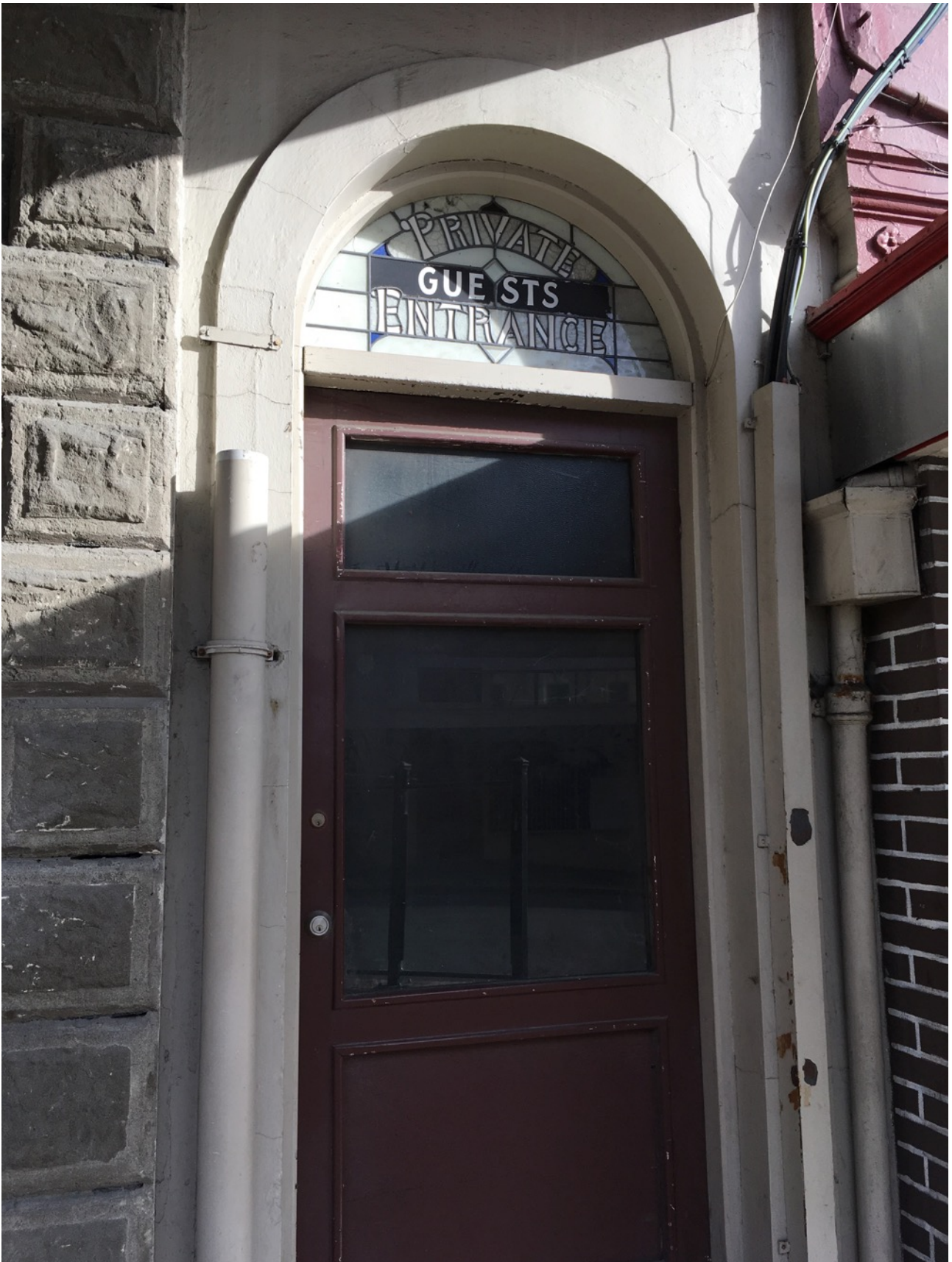
Guests' private entrance; the style of the fanlight suggests that the entry was part of the 1906 improvements to the building. A McEwan, July 2018.
