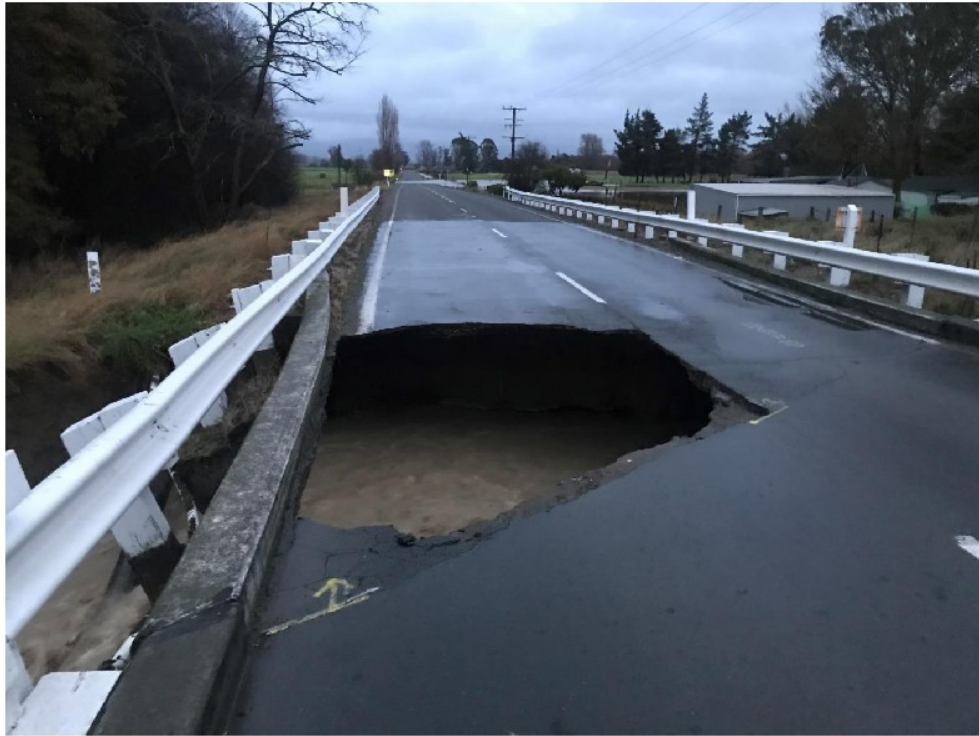
Waihi Bridge Damage
