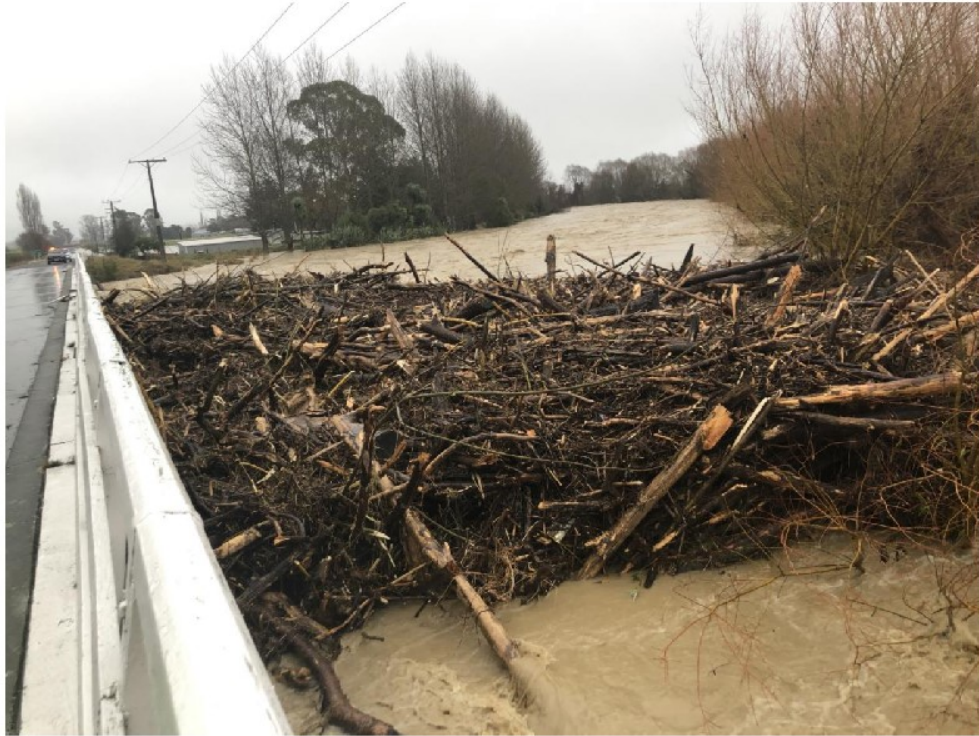
Waihi Bridge Debris
