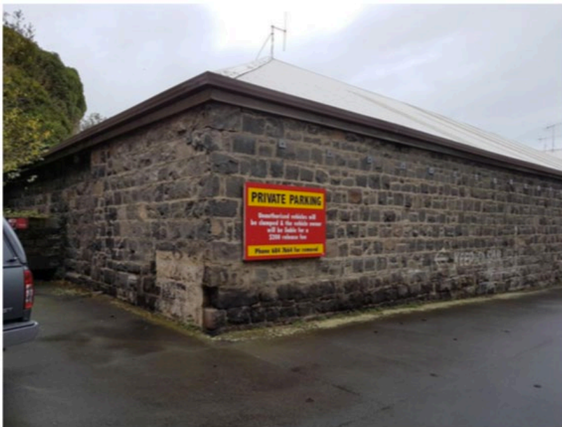
North-west corner of the bluestone block of the Pyne Gould Guinness Building (Former), R Burgess, 22 June 2017, Heritage New Zealand
