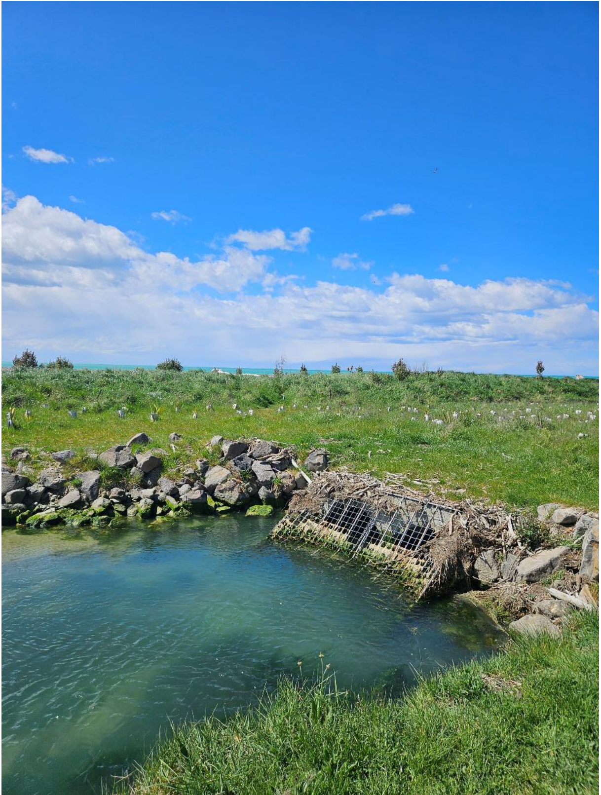
Figure I21: Washdyke Lagoon Ring Drain Coastal Outlet
