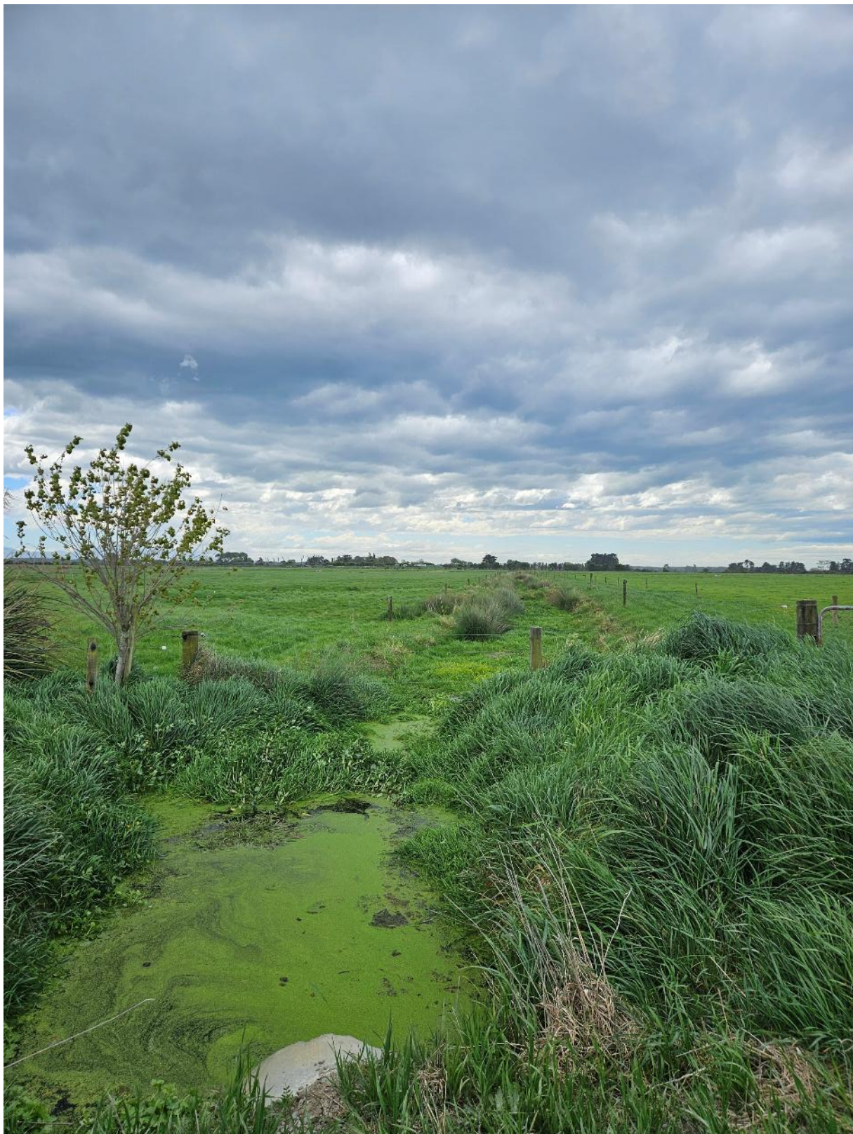
Figure I10: Beach Road Drain and Culvert, Connected to Philips Lagoon
