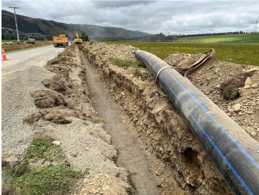
Te Ana Wai pipeline across Pahau Downs Road, working its way towards Eskdale Road.
