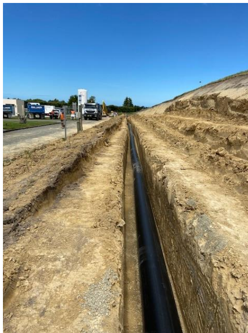
Contract 2470 – Pareora Pipeline Renewal Section 3 : Photo of pipeline being laid into the Claremont Reservoir grounds.
