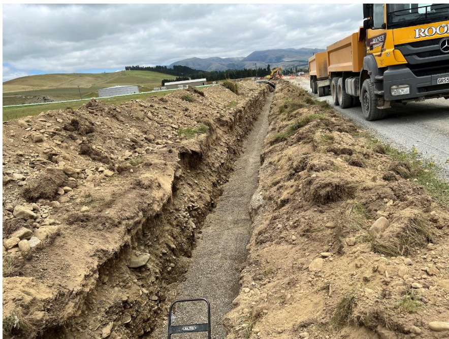
Te Ana Wai pipeline progressing (view of Te Ana Wai treatment plant and reservoir in background).
