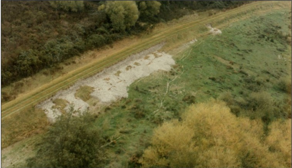
Figure 9-5: Opihi River stopbank on true right bank ~300 m upstream of Collett Road following overtopping during the 13 March 1986 flood
