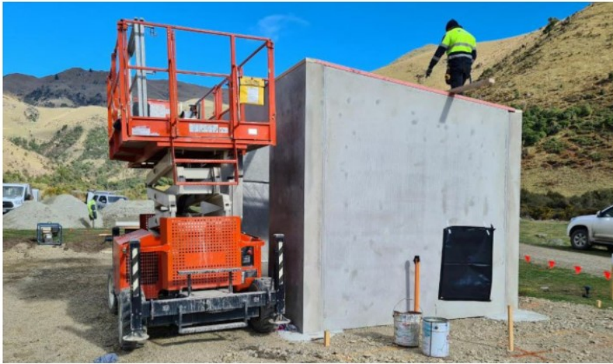
Contract 2468 – Flow Control Valve Station
