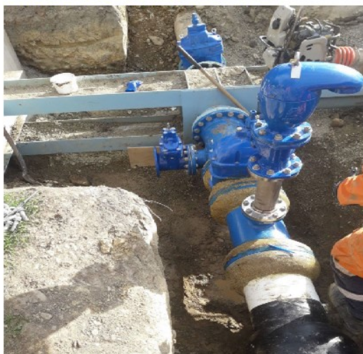
Contract 2338 - Te Ana Wai Pipeline Stage1 (Davisons Road to Cave) – Lining methodology
