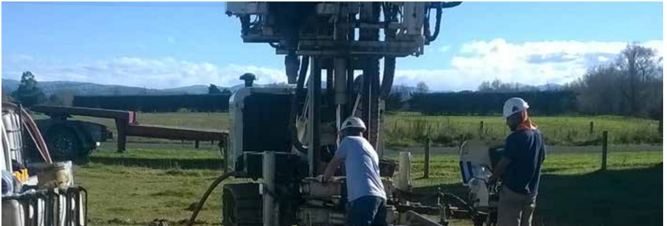
Temuka new bore, Temuka connection
