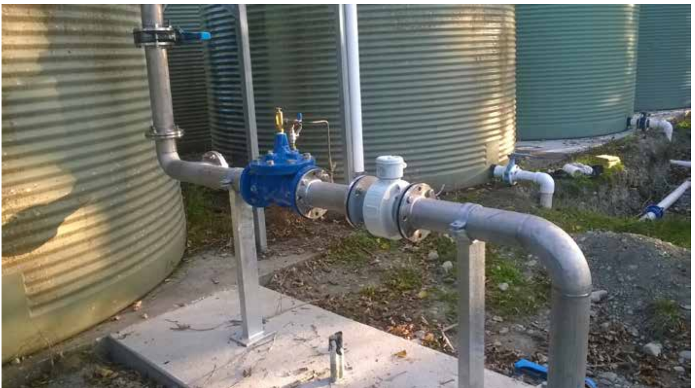
Additional water storage at Winchester
