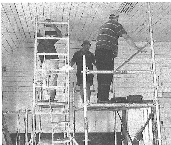
Hard at work - volunteers painting the ceiling of the Te Awa Rd hall.
