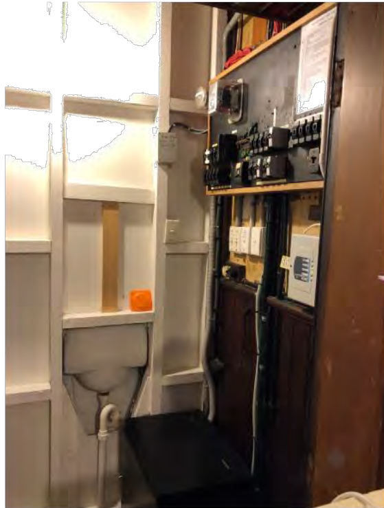
Figure 28 Space 13 electrical store
