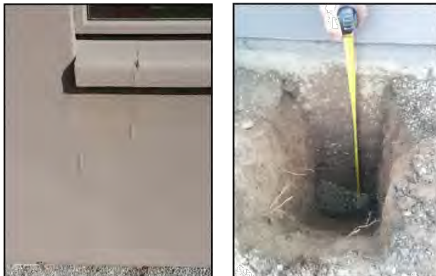
Figure 3: Photos showing the area along the northern side of the building (DCP4 location) where cracking of the block cladding was evident (left). Note the hand excavation below the area of cracking revealed drainage material, a PVC pipe and standing water. Photo taken 21/08/2019.
